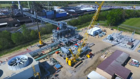
St. Mary Clean Energy Center
