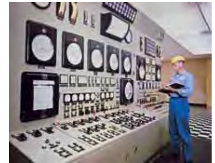
A worker monitors plant operation in the control room of the expanded Coughlin Power Station in the early 1960s.
