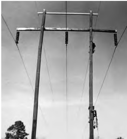
LEFT: Transmission lines like these made up the backbone of the Cleco system in the 1940s and 1950s.
