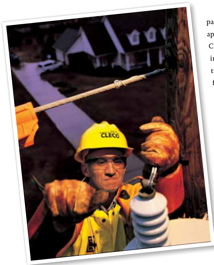
The basics are still important. David Feucht, lead line mechanic, repairs a residential transformer in the early 2000s.
